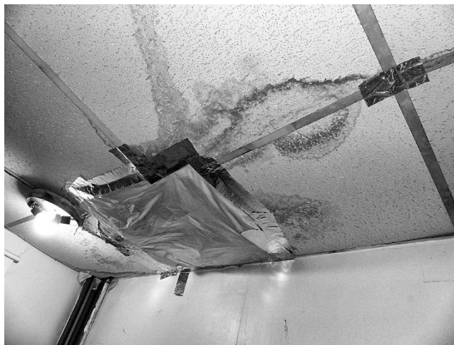
“Repair” of bathroom ceiling at 215 Wilson Street
