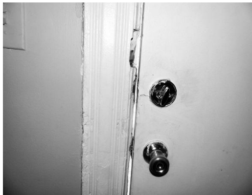
Unsafe and drafty apartment entrance at 163 Concord Street
