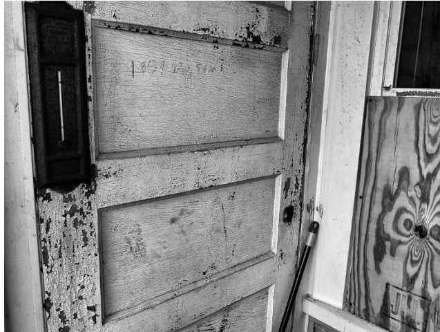
Flaking and peeling paint at 215 Wilson Street
