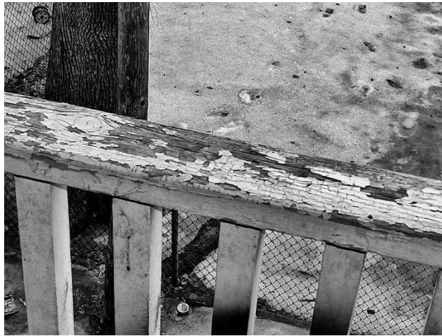
Flaking and peeling paint Concord Street MPBUH Holdings LLC
