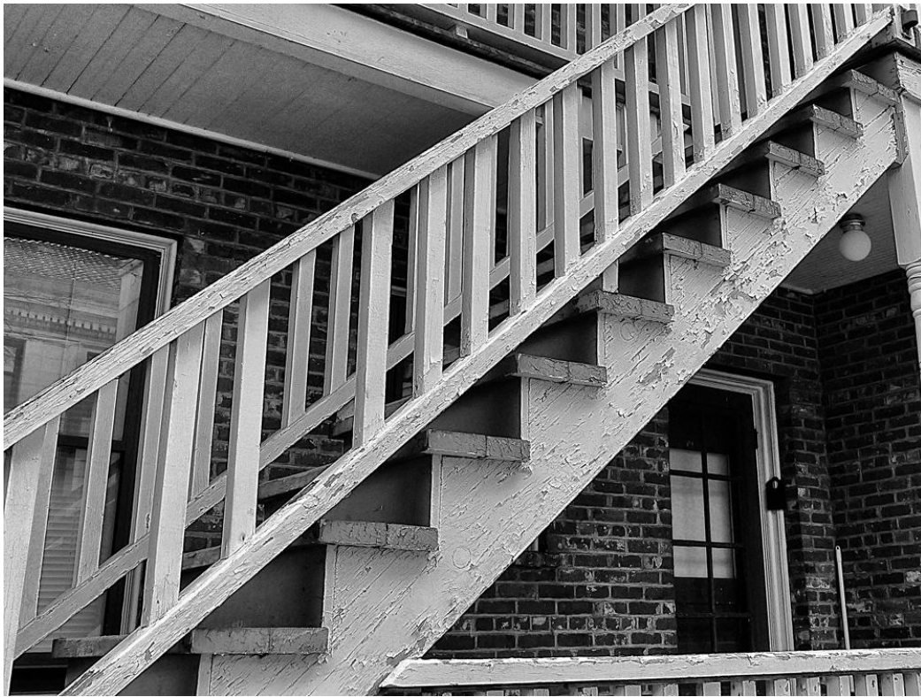
Deteriorating Lead Paint Concord Street (MPBUH Holdings LLC.)
