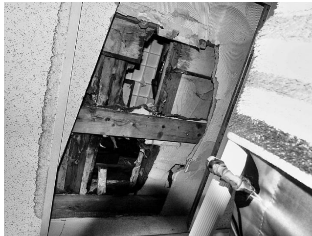
Bathroom ceiling at 205 Wilson Street
